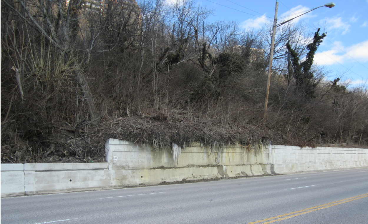
Figure 21: Toe of Landslide 8, 2019
