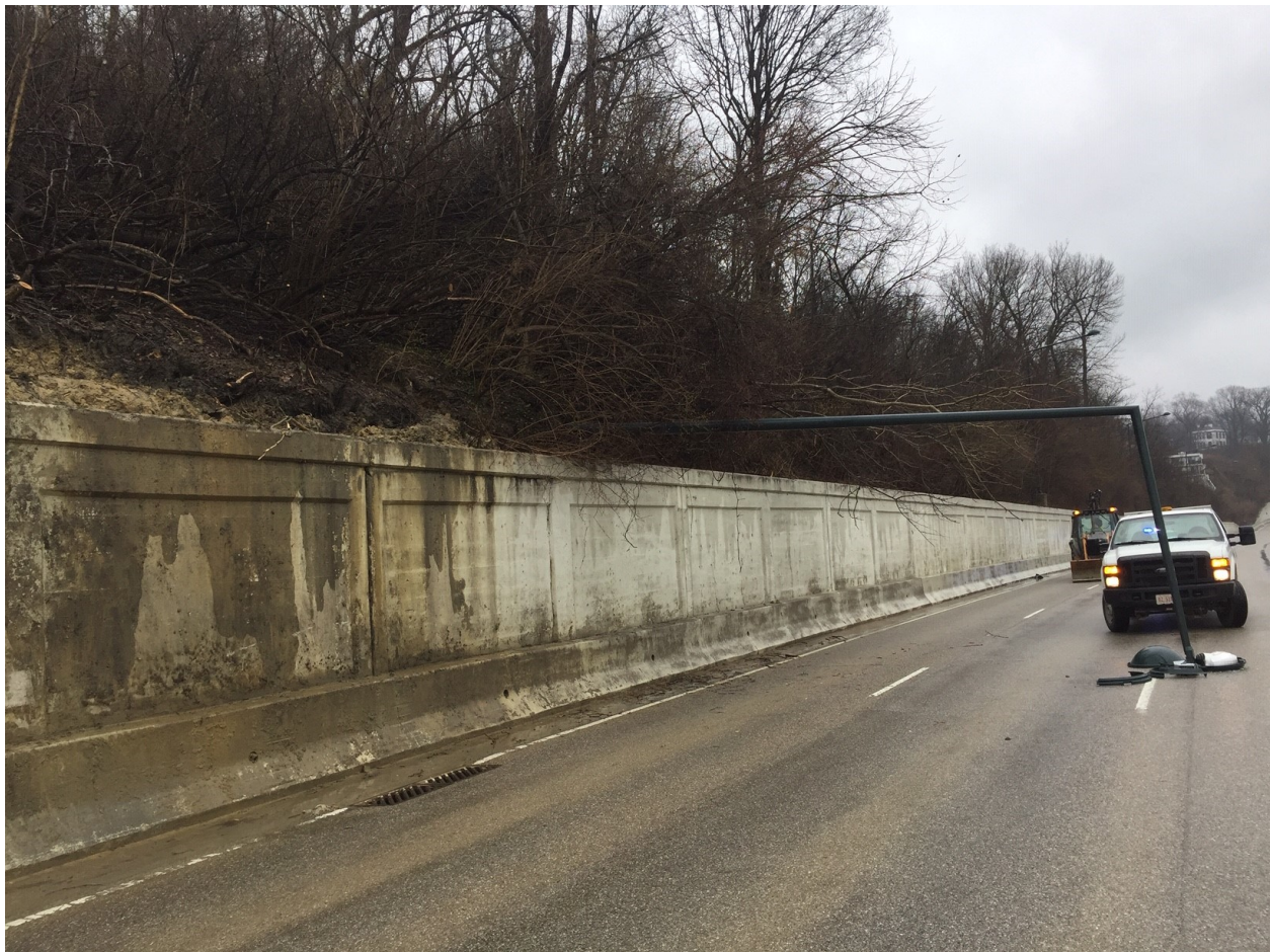
Figure 25: Landslide knocks over light pole, March 25, 2019
