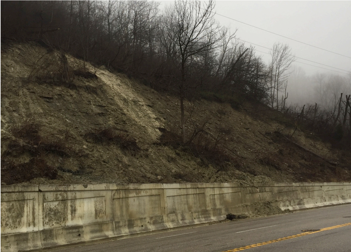
Figure 8: Feb. 11 th , 2019 debris coming over the wall 1,000 ft. east of Kemper Lane
