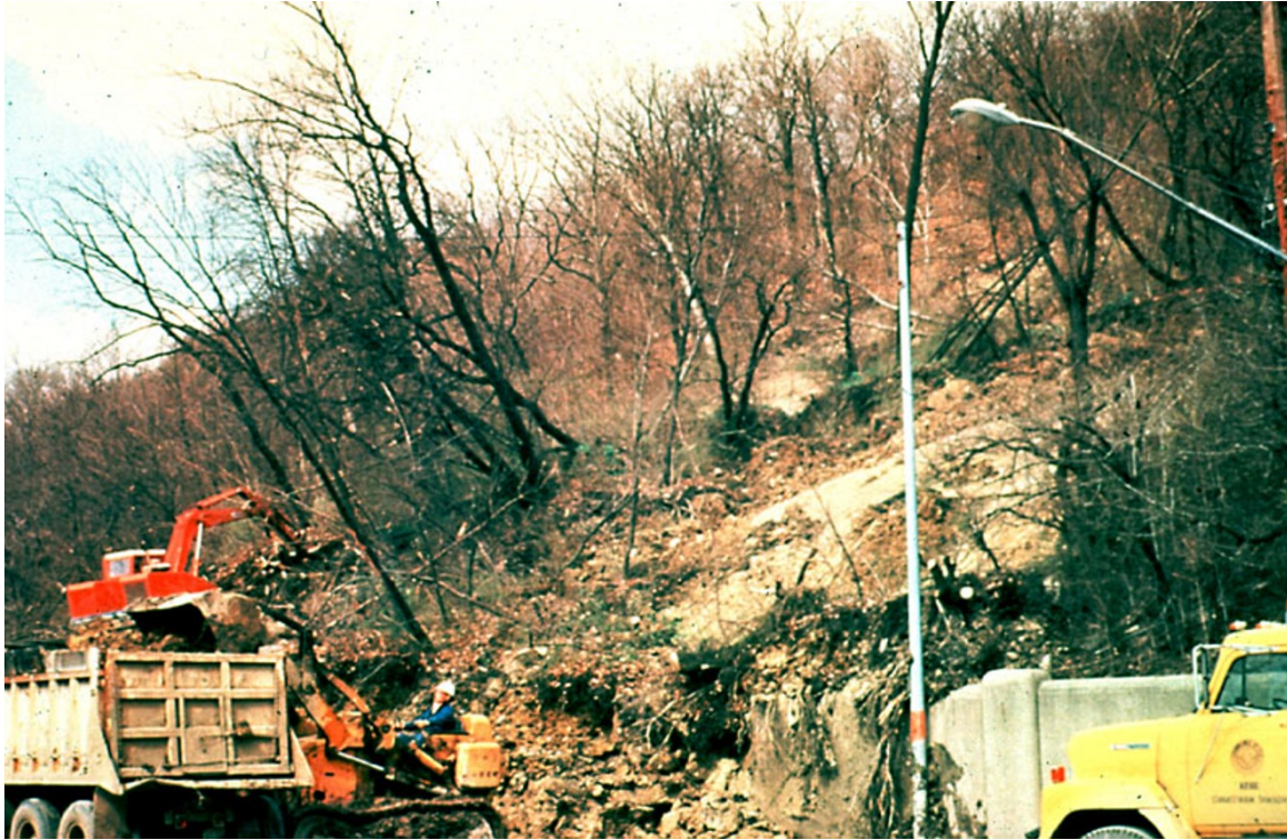
Figure 4: 1975 Landslide clean-up. U.S.G.S. Website
