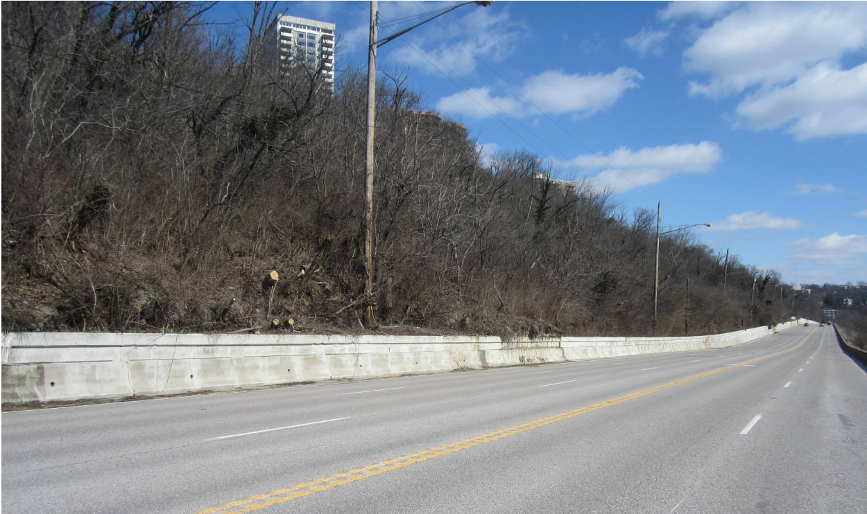
Figure 20: Toe of Landslide 7, 2019
