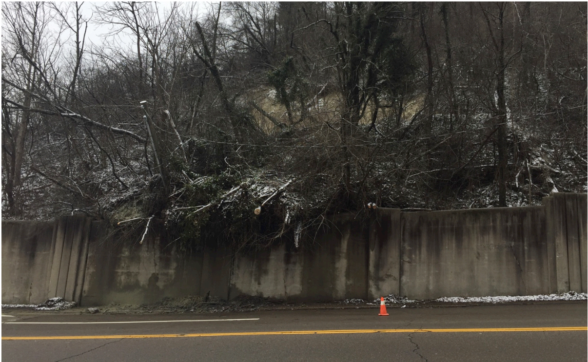
Figure 6: Jan. 24 th 2019 landslide on Kemper Lane
