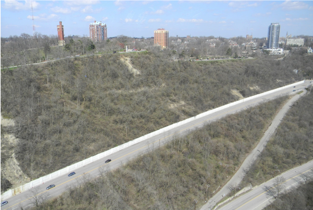
Figure 16: Landslide Areas 1 west, 2 & 3 2012
